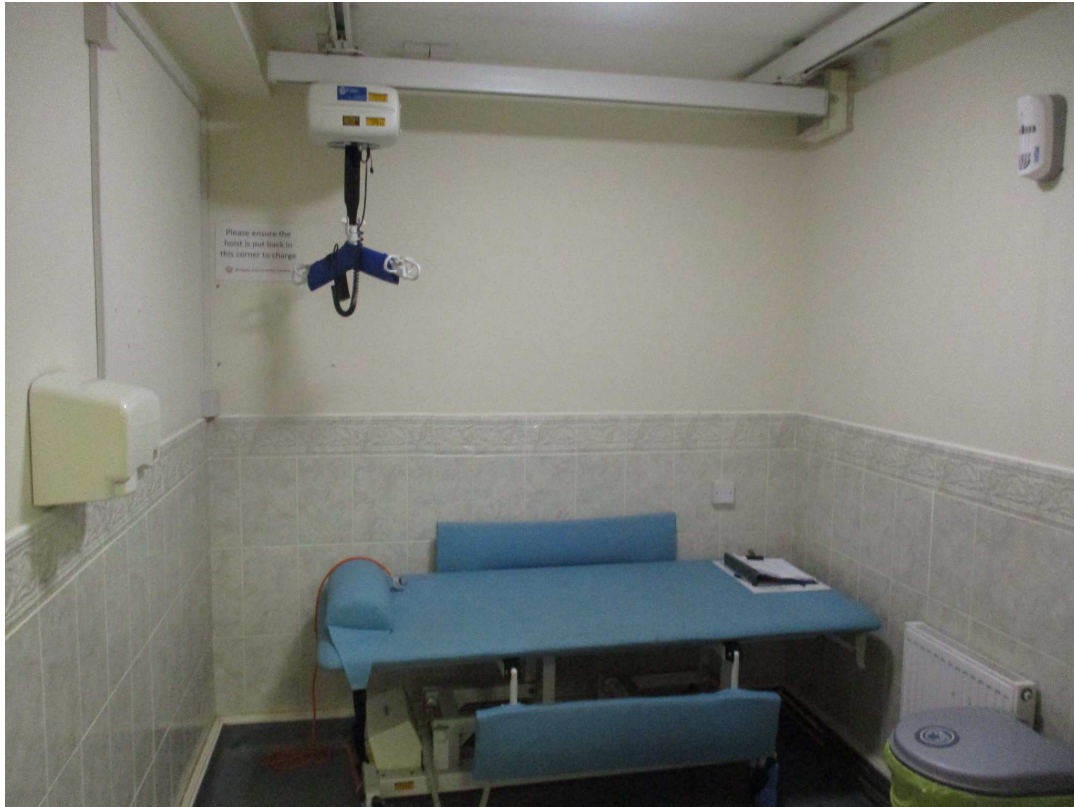
Photo 30 Existing undersized Changing Places WC.
