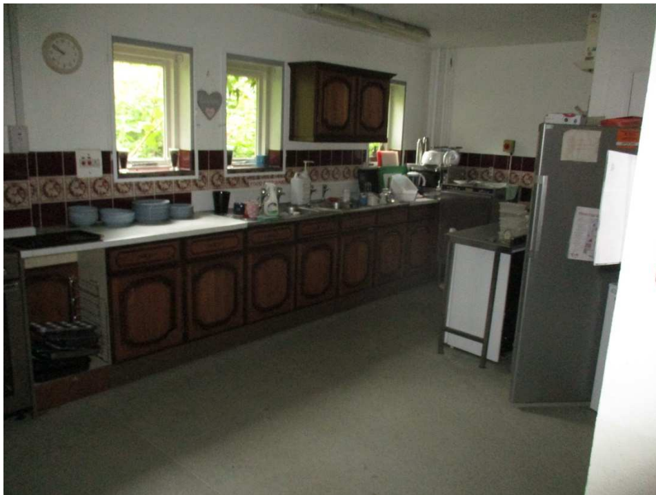
Photo 4 – Kitchen, no accessible facilities
