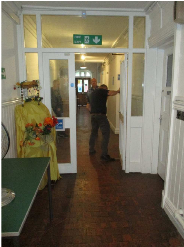
Photo 12 – Cross corridor door, not held open.
