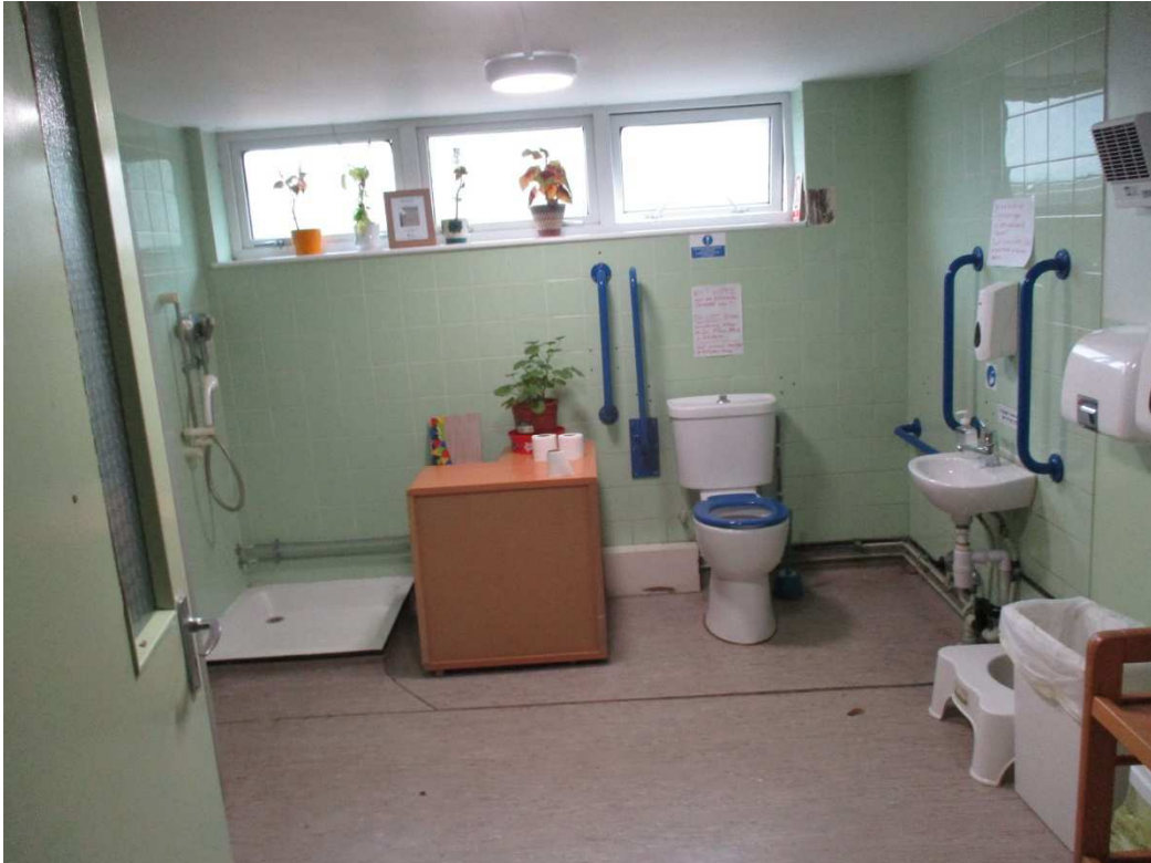
Photo 18 – Existing WC/ shower facility/ Proposed upgrade to Changing Places WC Low ceiling height will prevent install/ use of tracked hoist.
