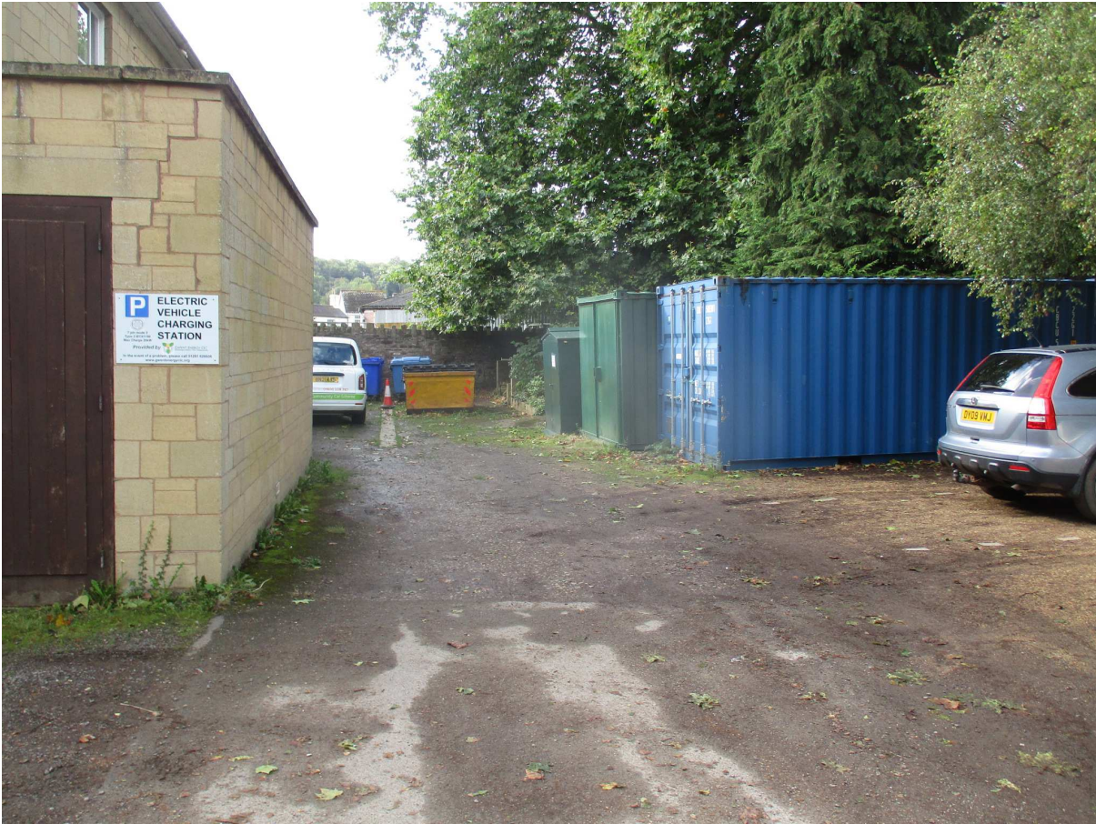
Photo 32 Uneven surfacing/ inadequate drainage on route from fire exit.
